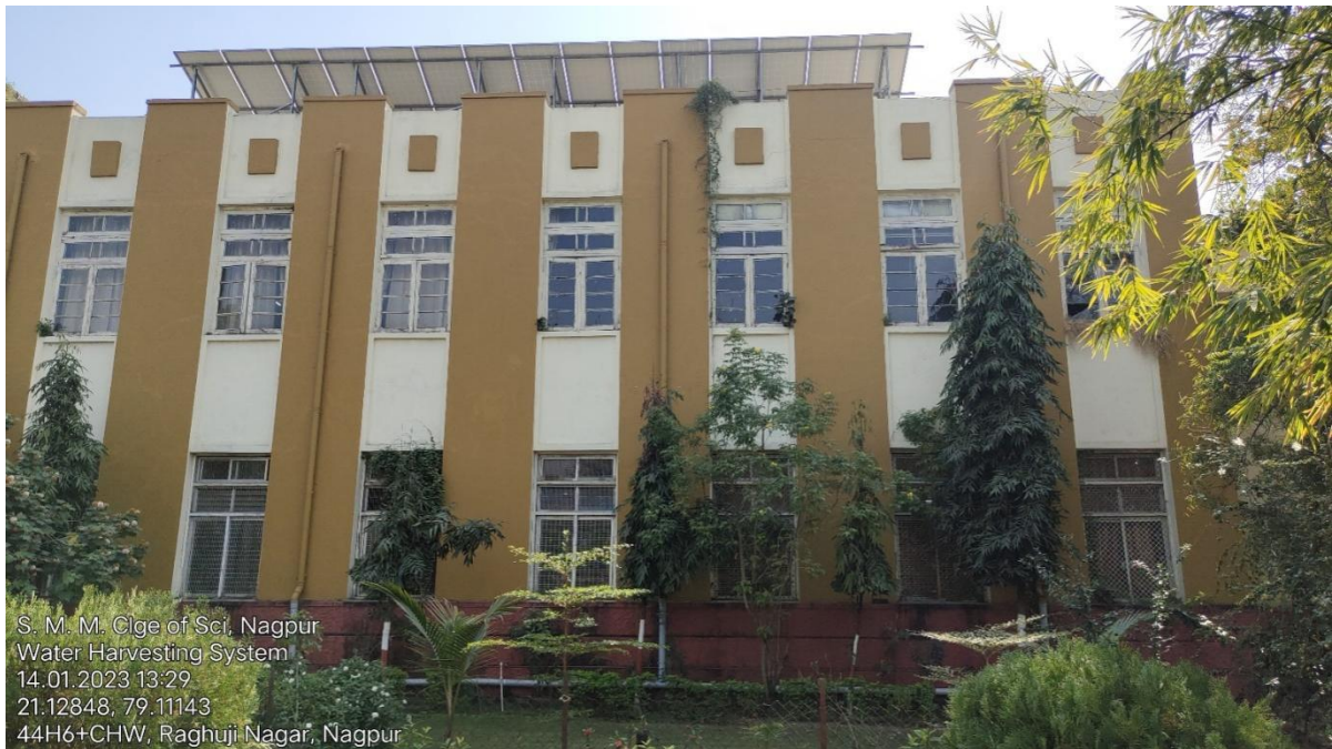
Pipes from the terrace bring water to FPS
