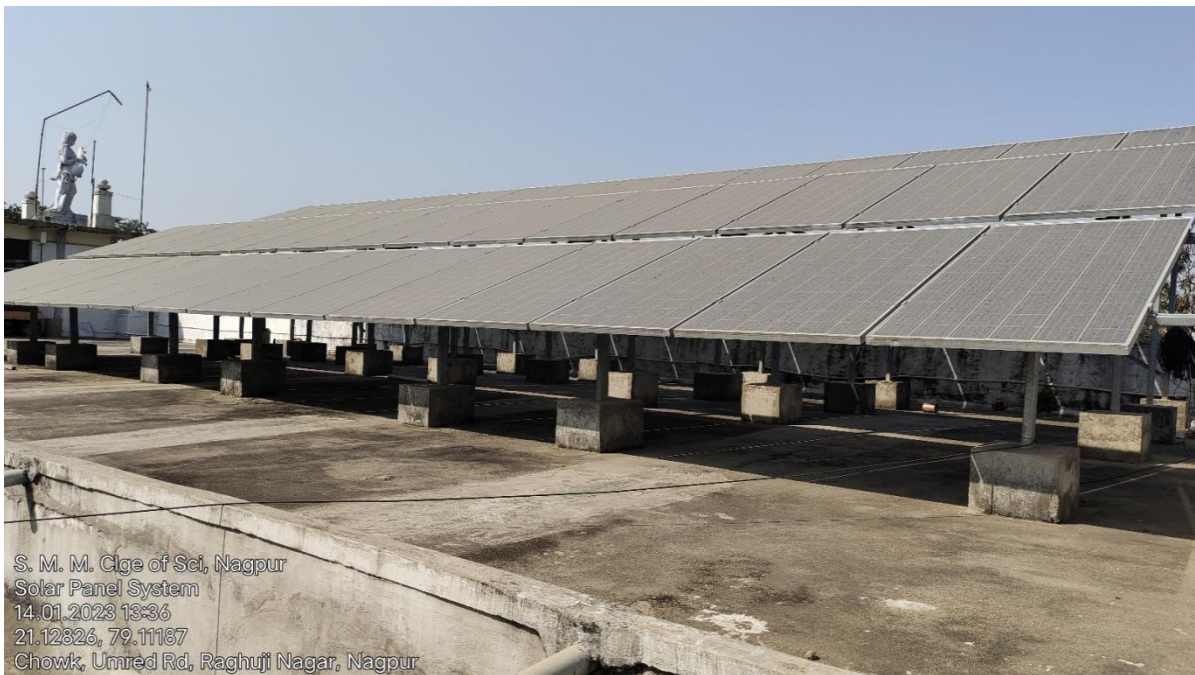
Solar panels Installed on both sides of terrace
