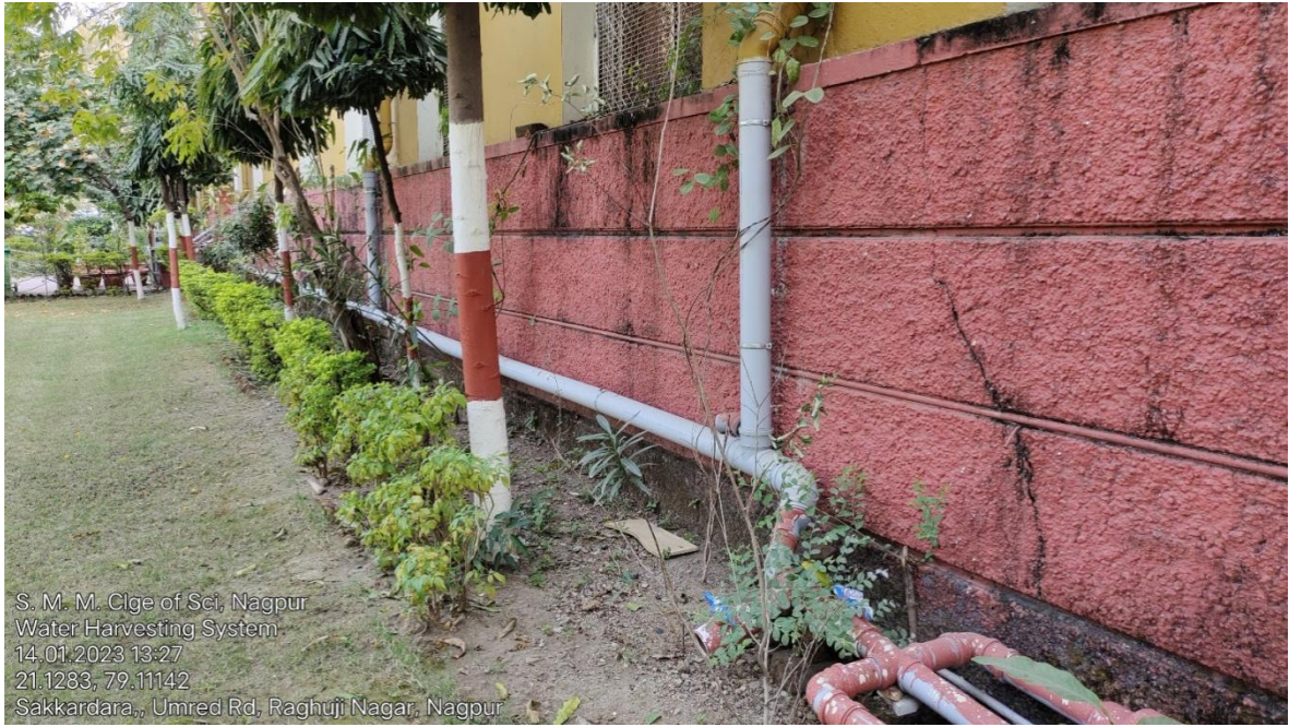
Pipes from the terrace bring water to FPS
