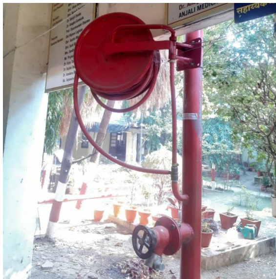
Fire fighting system installed in the college
