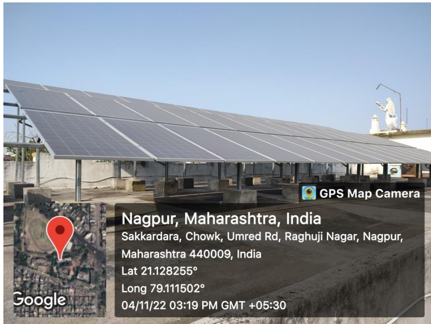
Rooftop solar system in the college
